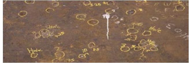
CORRODED PLATE SAMPLE Extensive top side corrosion pitting.
